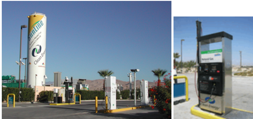
Figure 4. Public fueling at SunLine's Thousand Palms CNG fueling station
