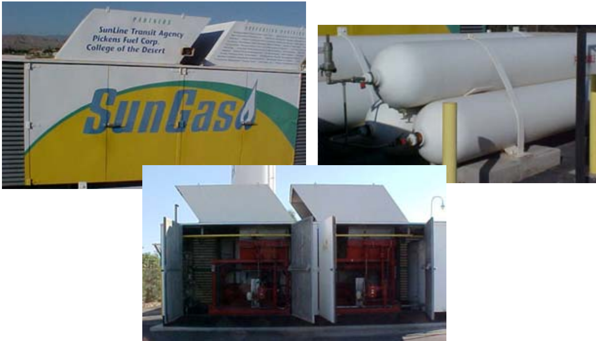
Figure 6. CNG compressor station (Thousand Palms)
