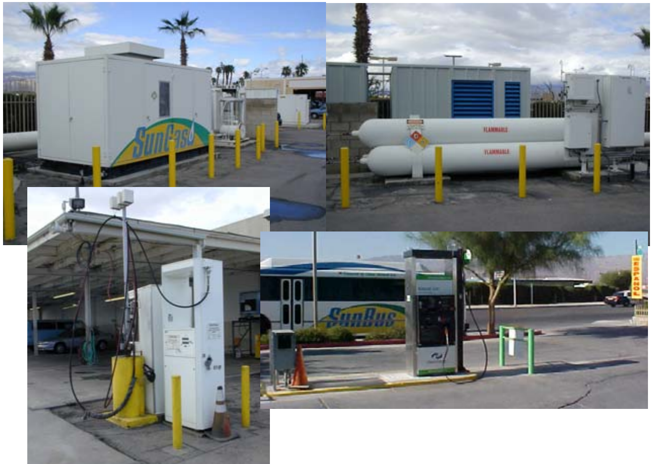
Figure 8. CNG fueling equipment (Indio)
