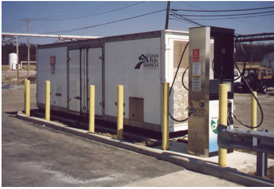
Figure 1. On-Site CNG Fueling Facility
