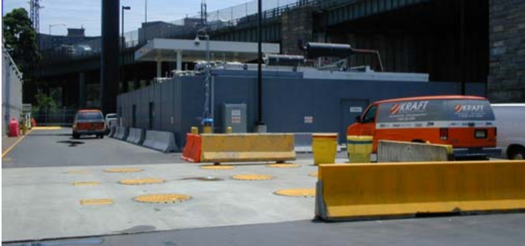
Figure 4. CNG Compression Station at West Farms Depot
