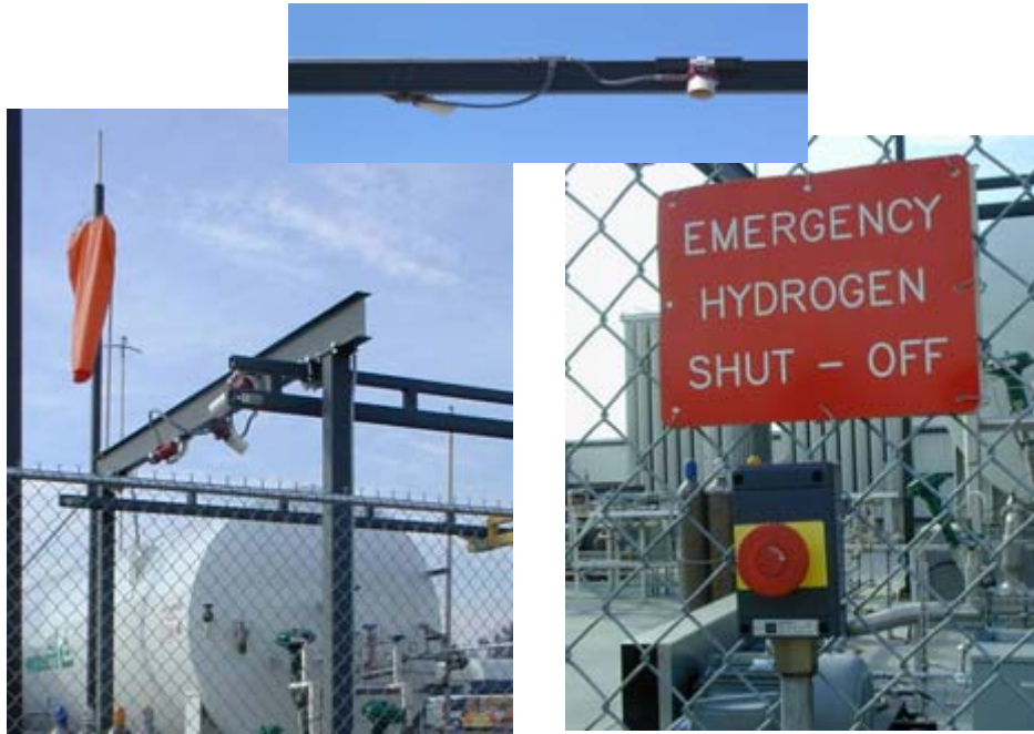
Figure 5. Flame Sensors (left and top) and Emergency Shut-off (right) at the Hydrogen Dispensing Facility
