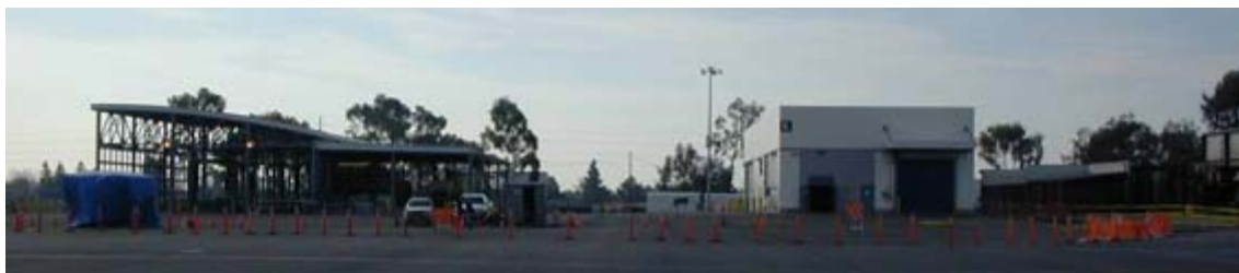
Figure 10. Bus Wash (left) and Maintenance Facility (right)
