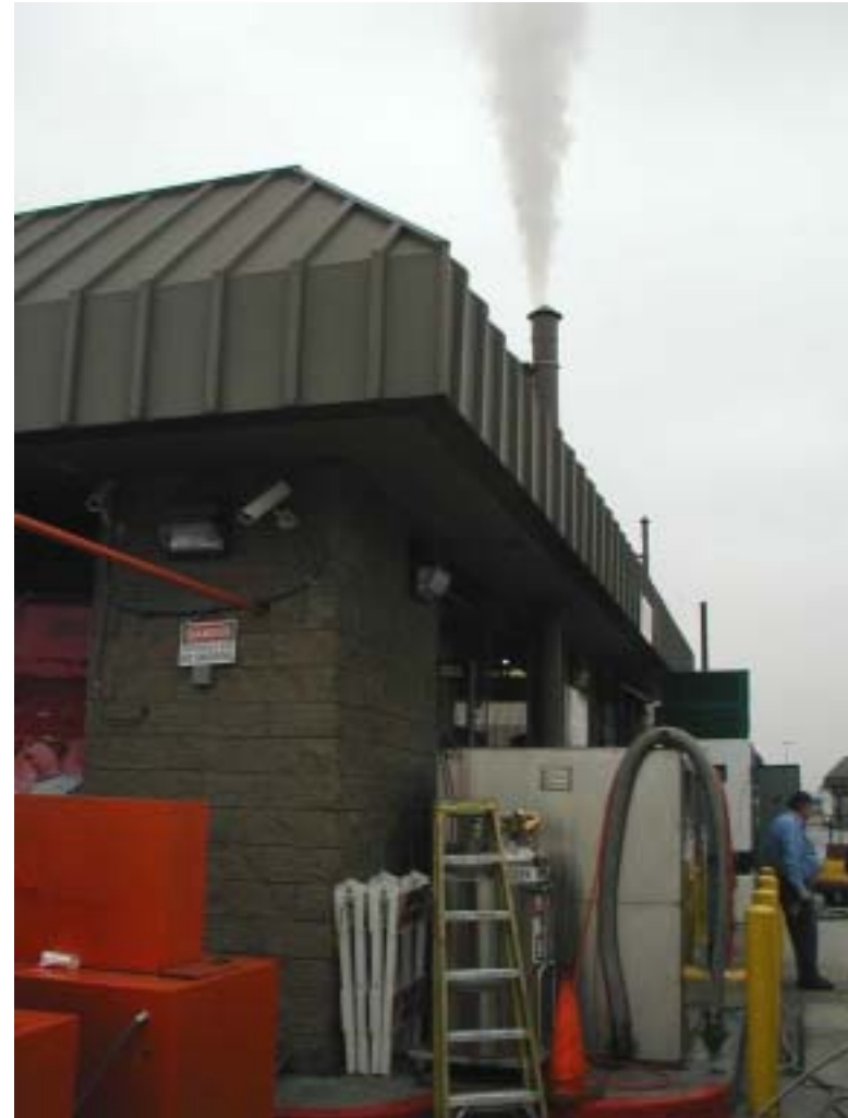
OCTA's Garden Grove LNG Station Venting Methane
