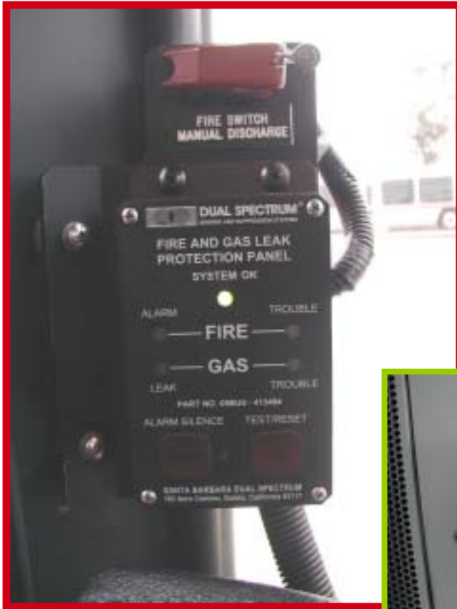
Driver's fire safety panel
