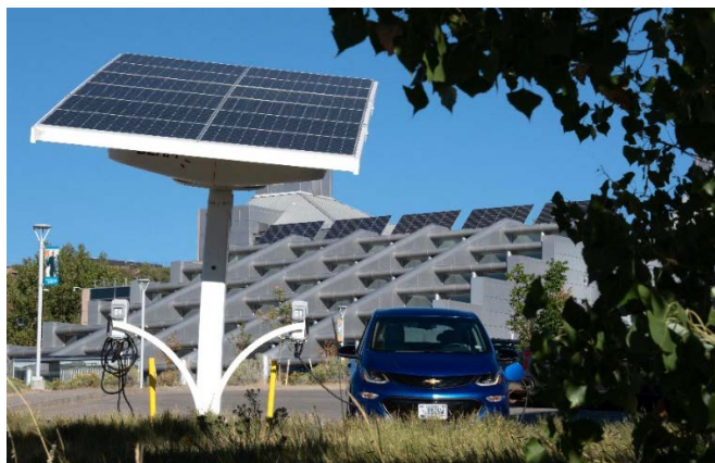
Figure 11. Solar EV charger on the NREL campus.
