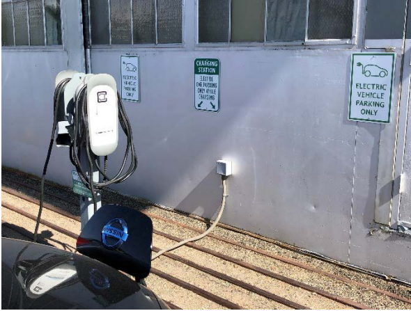
Figure 9. A Nissan LEAF plugged in at a charging station.
