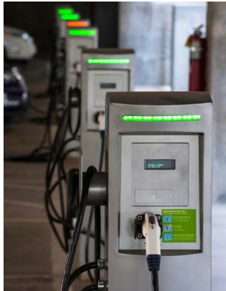
Drivers of EVs and PHEVs have access to thousands of charging stations across the country. Photo by Dennis Schroeder, NREL 22658
