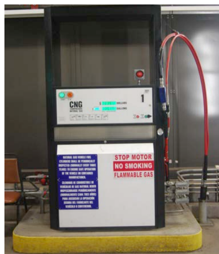
Figure 5. Glenwood Maintenance Facility indoor CNG fueling pump. Photo by George Mitchell, NREL 34977
