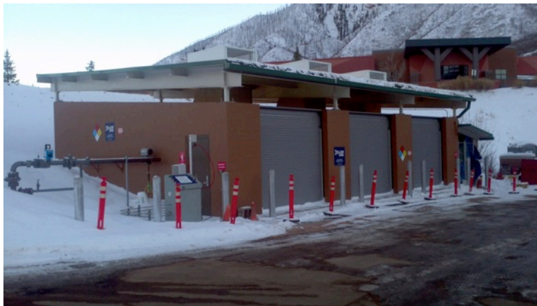
Figure 3. RFTA's CNG compressor station and de-fueling facility. Photo by George Mitchell, NREL 34978
